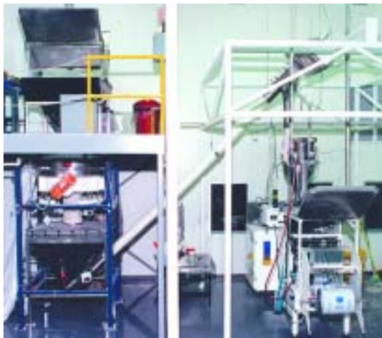
On-size powder is discharged from the Kason screener through a floor hopper into a flexible screw conveyor that transports the powder through an interior plant wall to a filler and vertical form-fill-seal packaging machine in the adjacent room.
