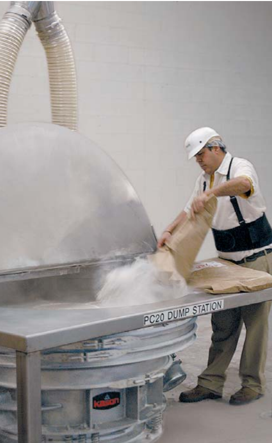
Caravan Ingredients built this bag dump station, which incorporates a stainless steel platform table, a 60 in. (1524 mm) diameter low-profile vibratory screener from Kason, and a dust collection system.
