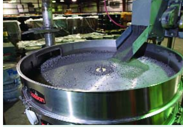
A view of the top of the separator and the feed chute from a different angle. The port through which large particles of ferrotitanium are removed is at the upper left.
