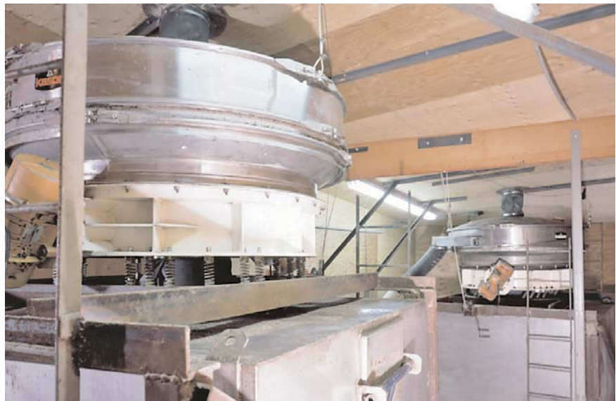
Two 72" (1829mm) diameter Kason low-profile Flo-Thru Vibroscreen® circular vibratory separators are mounted on holding bins that discharge urea, phosphates and potassium granules into bagging machines below. Screeners prevent separation of ingredients having disparate bulk densities to produce a uniform fertilizer product.
